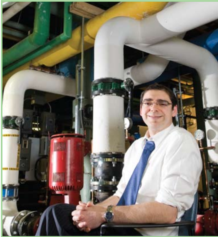
Michael Boudana in the boiler room.
