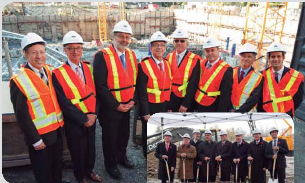
From left: Irwin Cotler, Rick Dubrovsky, Pierre Arcand, Lawrence S. Bergman, Dr. Hartley Stern, Dr. Yves Bolduc, Hai Pham-Huy and Philippe Castiel at the Pavilion K construction site on October 7, 2011.
